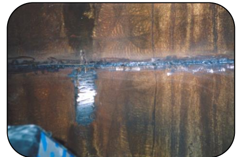
Damaged tank seams filled and rebuilt using 102 Metal Repair Fluid
