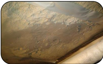
Base of tank, plate bonded and then resurfaced using 102 Metal Repair Fluid.
